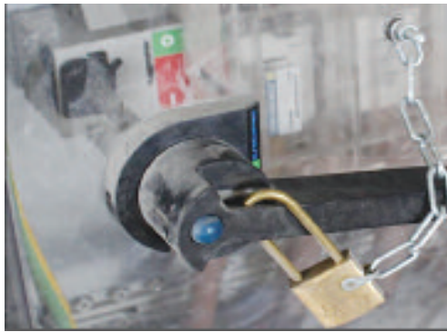
Fig 11.1 Electrical supply isolated and padlocked "off"
