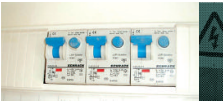
Fig 7.1 Residual Current Devices (RCDs) (fitted to protect socket circuits)
