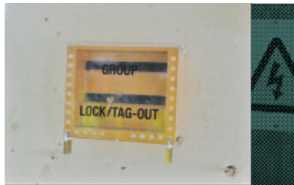
Fig 11.2 (a) and 11.2(b) Alternative procedure for ensuring safe isolation. Key of isolator padlock locked in cabinet with operatives personal padlocks
