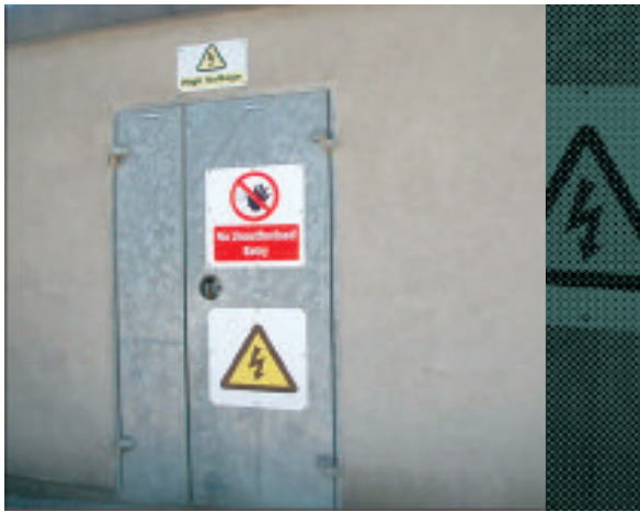
Fig 6.1 Access controlled to high-voltage switch room
