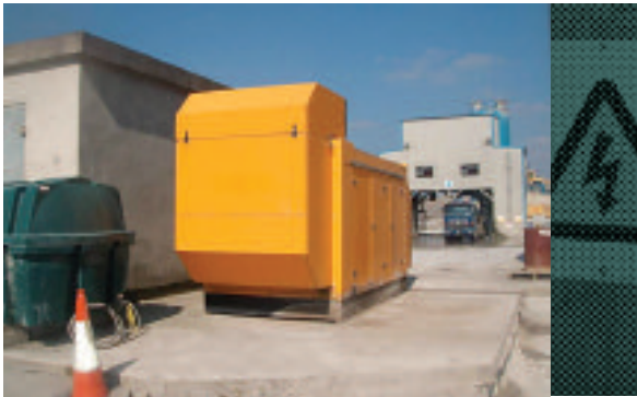
Fig 10.1 Emergency generator Installation (To maintain electrical supply in the event of a power cut)
