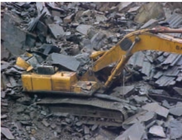
Figure 4: Crushed by Face Collapse
