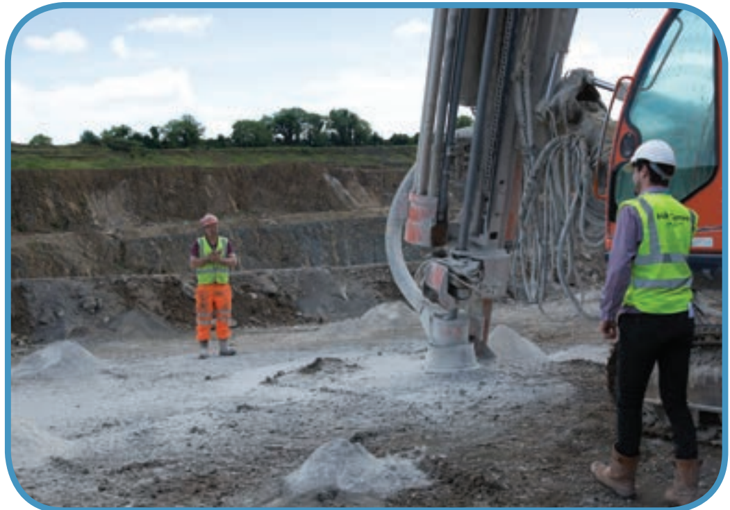
Quarry Workers marking out drill holes with fall protection provided by bunded edge protection made from quarried material
