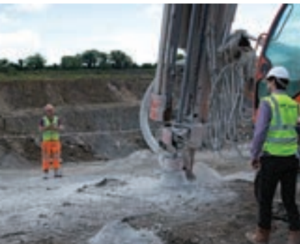
Figure 28: Face Edge Bunding system in Operation
