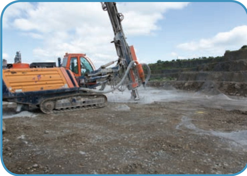
Drill Rig Operator working at a Quarry Face with fall protection provided by bunded edge protection made from quarried material
