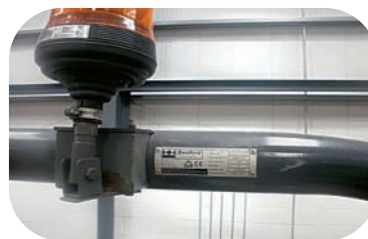
Identity plate on ROP's showing CE mark
