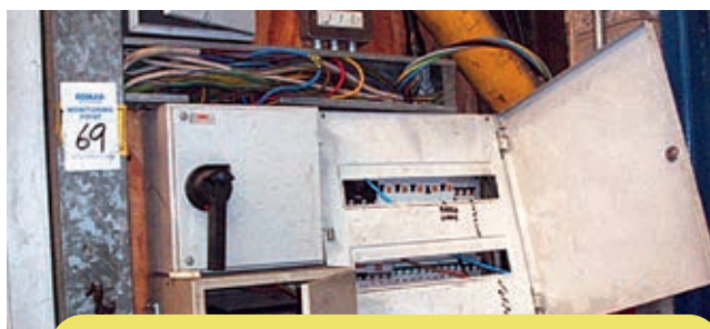
Fig 7.4 Installations like these can lead to inadvertent contact and electrocution
